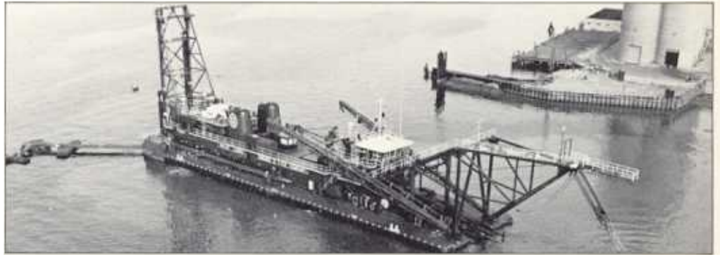
The hydraulic dredge is excavating a trench in the harbor bottom for the tunnel.
