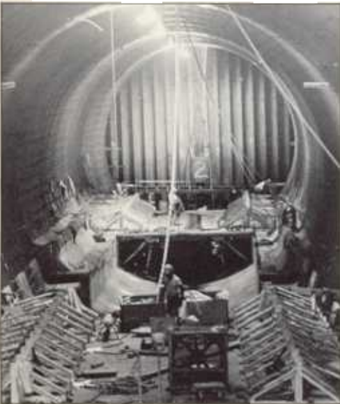
At the outfitting pier, near the tunnel site, concrete is added to interior and exterior portions of the tubes.
